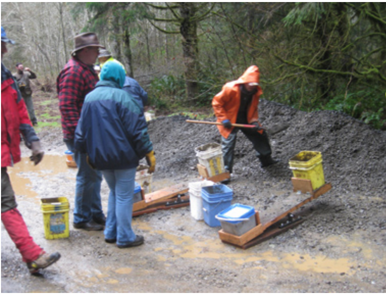
Great Gravel Pack-In March 29th. Loading buckets using the makeshift scale to be sure the buckets weigh the same.
